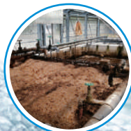
Wastewater treatment tank (aeration)
